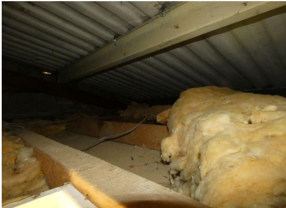
Photograph 10: Poorly distributed insulation in the roof void.
