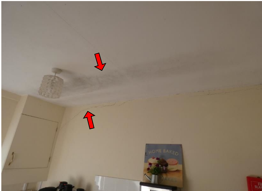
Photograph 11: Condensation mould to the kitchen ceiling and crack to the rear left-hand corner.
