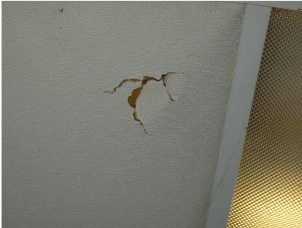
Photograph 9: Damaged tile to the factory lining system.
