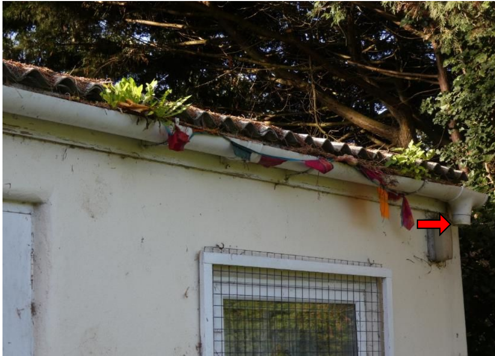
Photograph 7: Leaves accumulating on the roof and in gutters. Note missing front right-hand rainwater downpipe.
