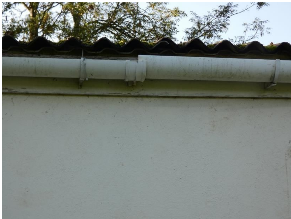
Photograph 12: Defective joint to the front rainwater gutter.
