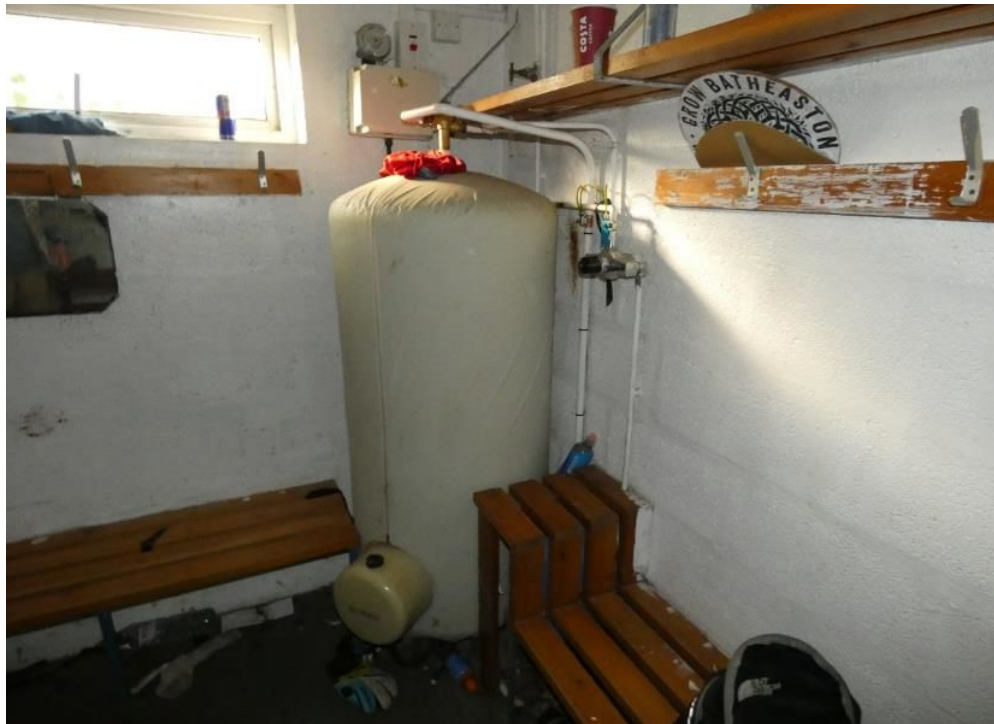
Photograph 16: Hot water cylinder to the changing rooms.
