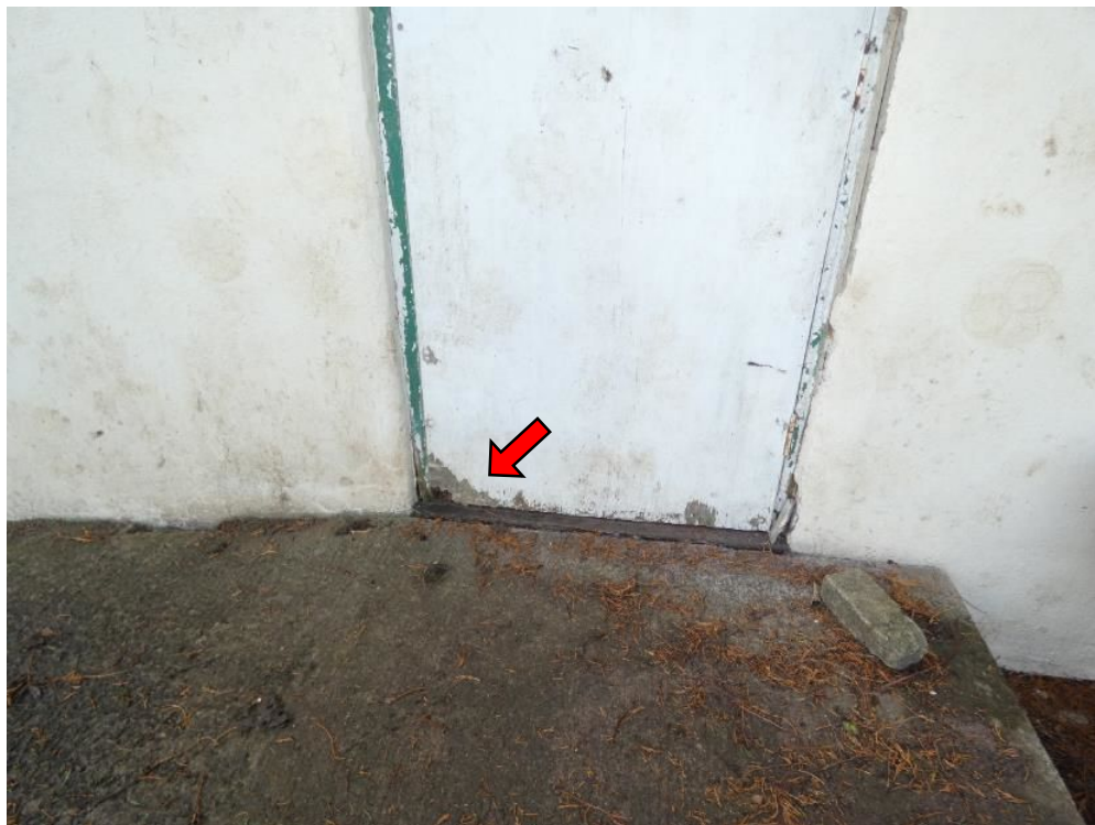
Photograph 14: Rot to the base of the front right-hand door.
