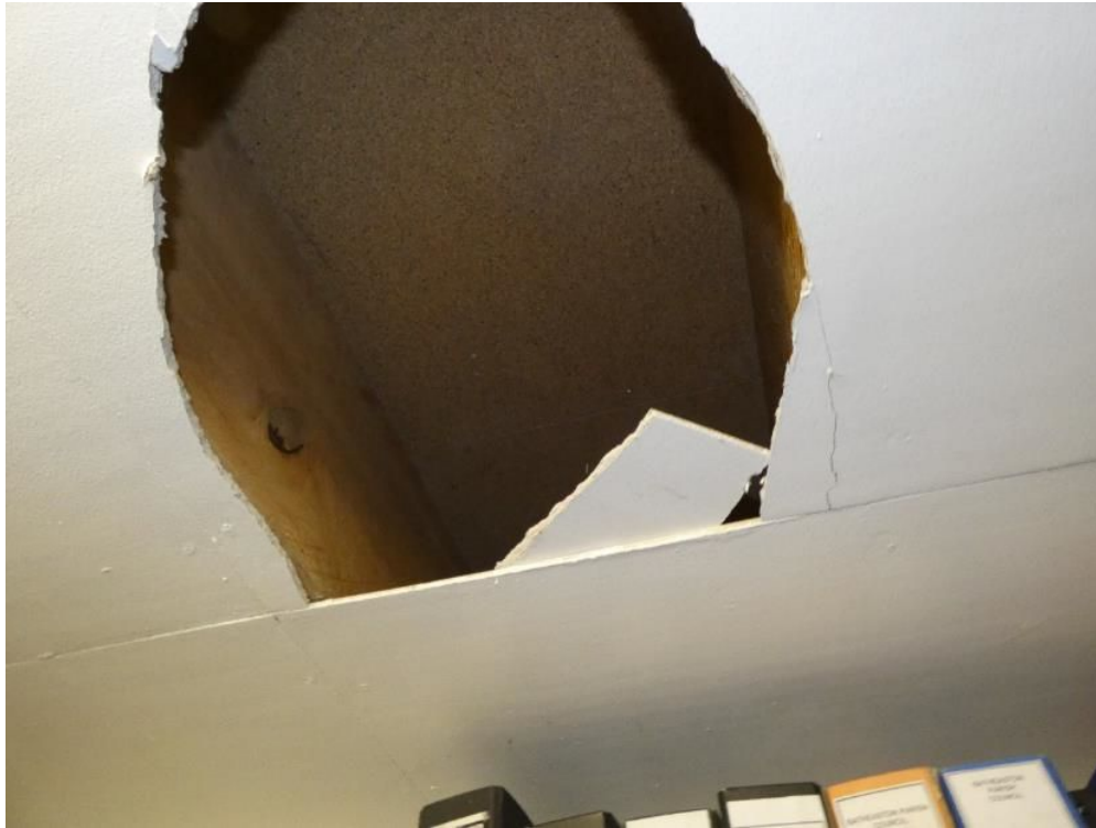
Photograph 15: Hole in the cementitious ceiling board to the changing rooms.
